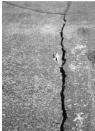
▲ Open crack – 1/2" or more in width.
