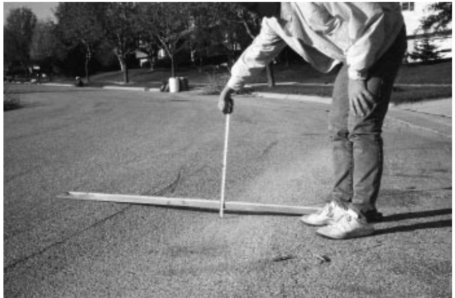
► Severe settling from utility trench.
