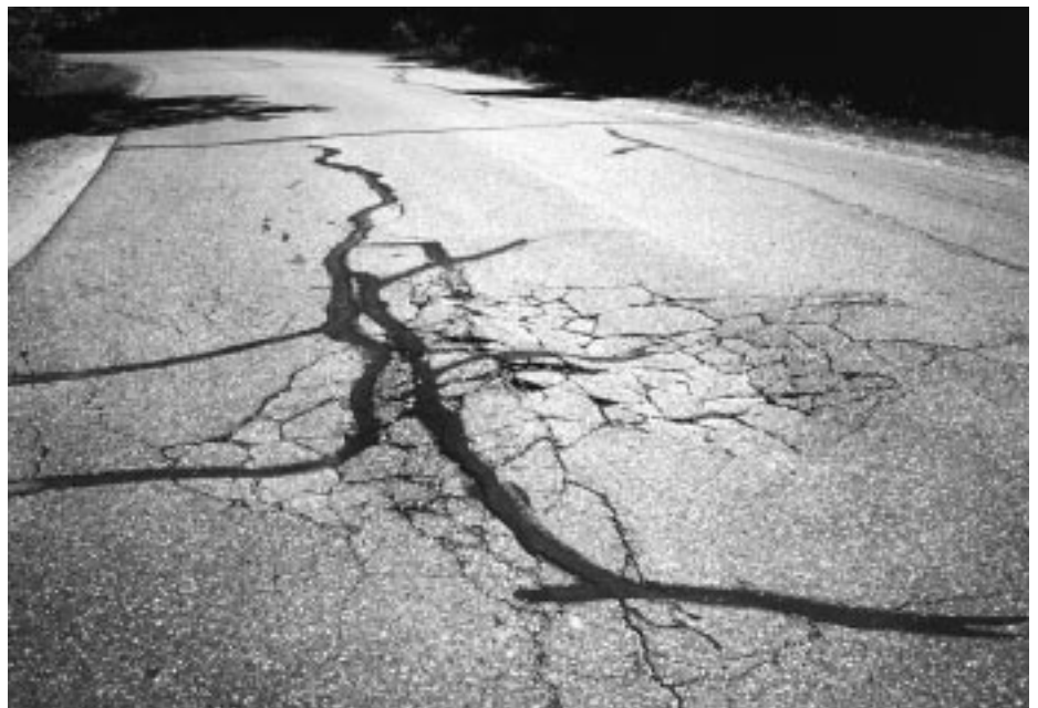
► Frost heave damage from spring break-up.
