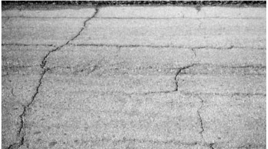
▼ Block cracking with open cracks.
