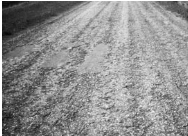
◀ Severe raveling and loss of surface material.
